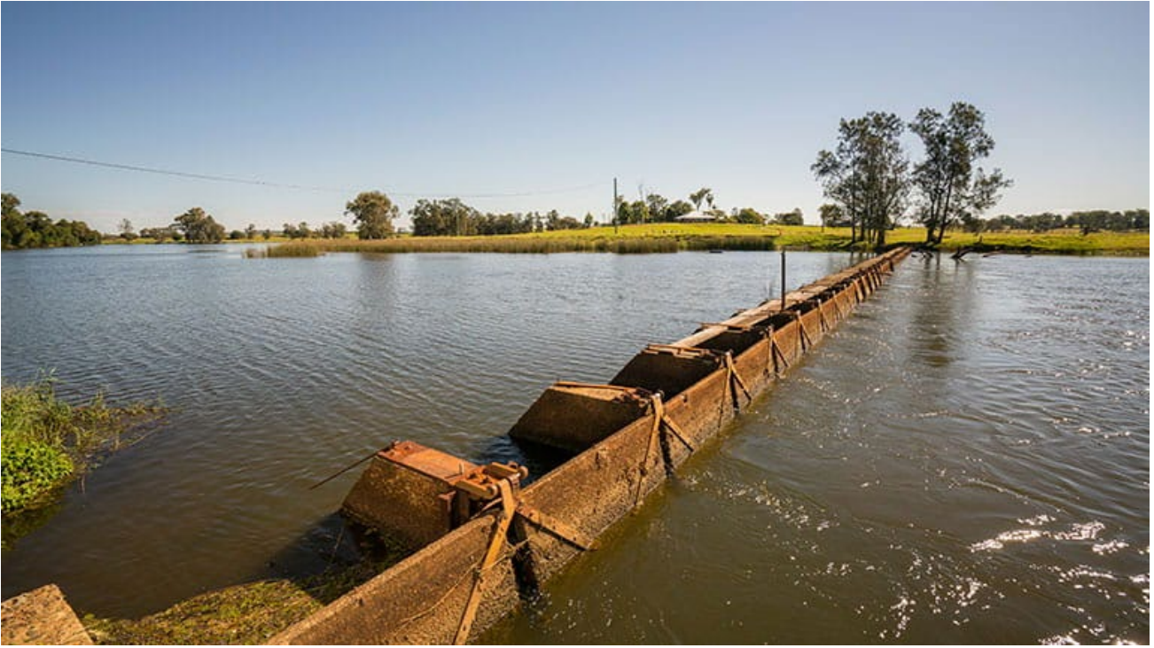
Figure 1. Sportmans Creek Barrage above the confluence of the Clarence River and Sportmans Creek (Photo NSW NPWS).
