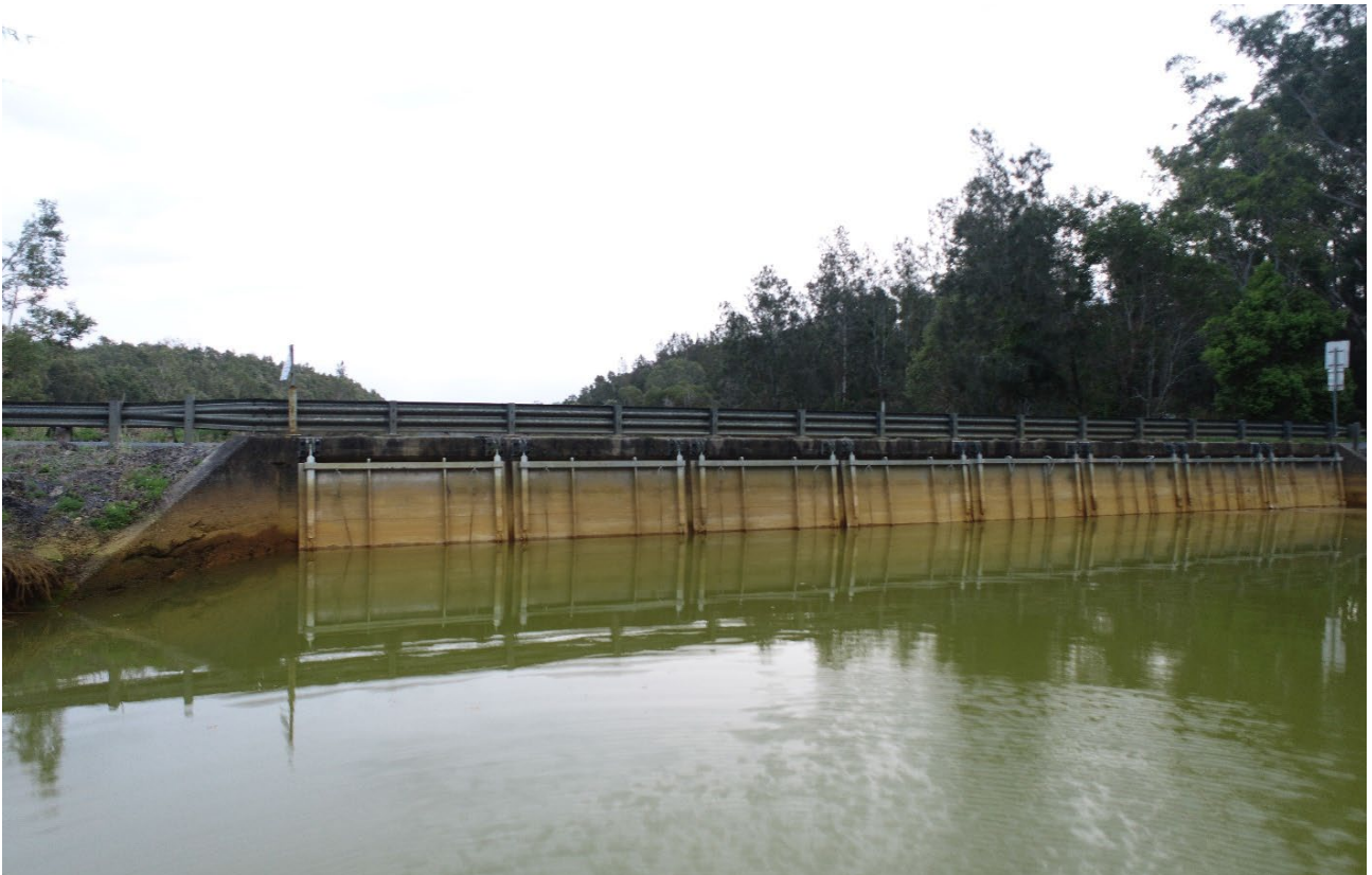
Figure 2. Tuckean (Bagotville) Barrage above the confluence of the Richmond River and Tuckean Broadwater.
